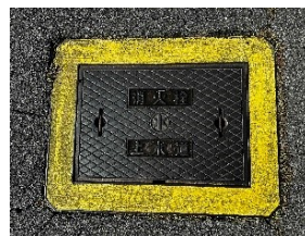
消火栓 (A hydrant)
